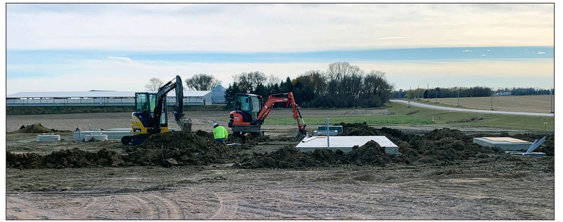
Mavis Fodness photo/1114 New Hills Substation
